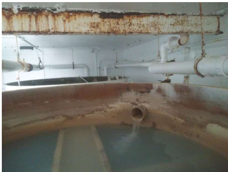
Image 2B: Corrosive Damage in Filter at North Plant
